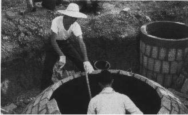
Figure 6: Installation of a Shanghai fixed-dome system near Shanghai, PR China Floating-drum plants
