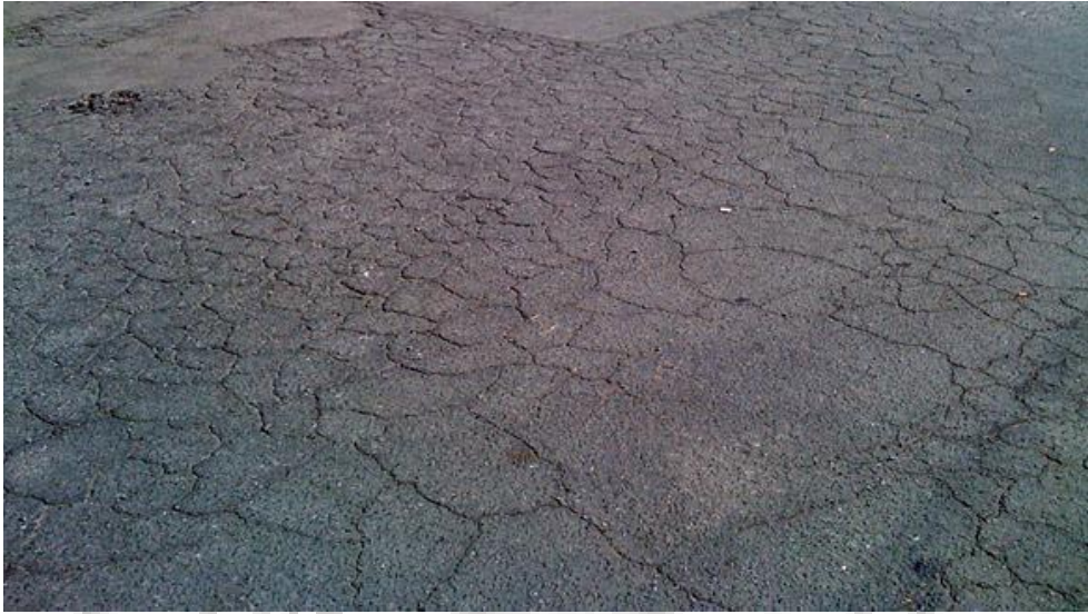
Fig. Alligator Cracking
