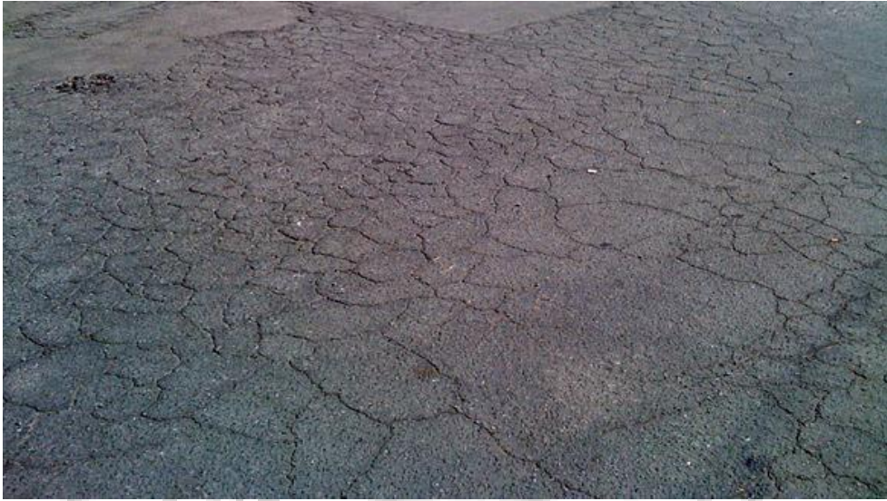
Fig. Alligator Cracking
