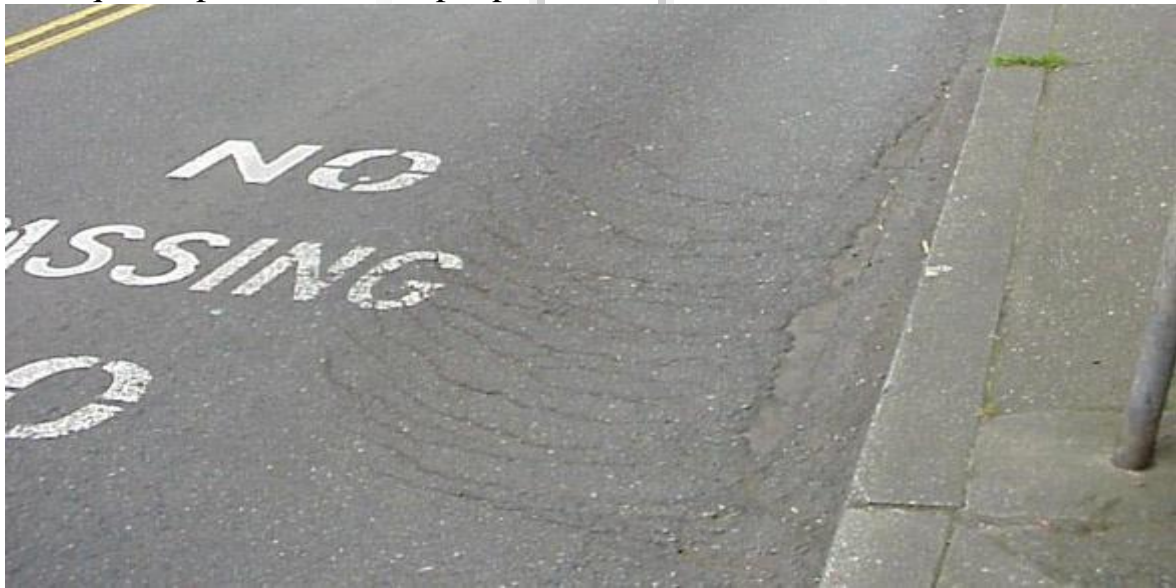
Fig. Slippage Cracks
