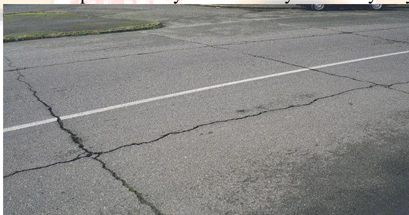
Fig. Joint Reflection Cracks
