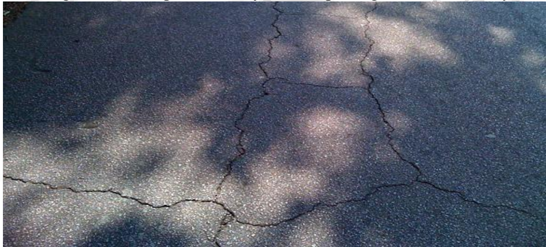
Fig. Block Cracking
