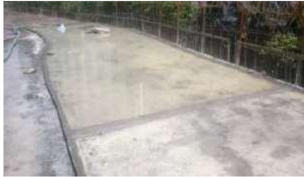
Fig:16 Ponding of slab
